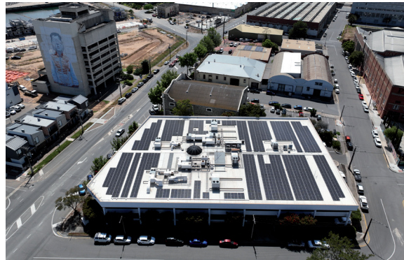
648 Solar panels supplying total annual power generation of 329,045 kWh to FPH head office.
